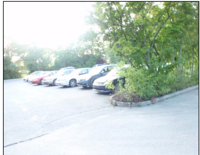
Surface pavement cracks and depressions.
